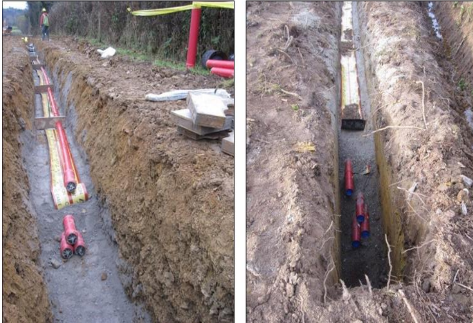
Plate 4-9 Typical Cable Trench View
